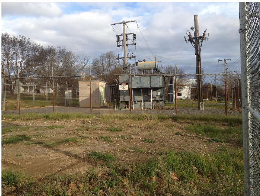
Photo 13: Existing substation which can be relocated
